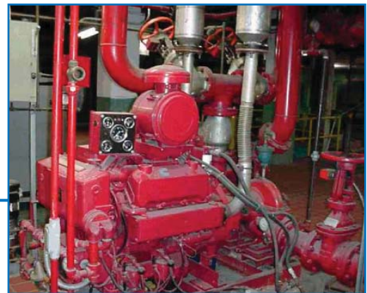
An existing fire pump retrofitted with an Armstrong Fire Pump Monitoring System.
